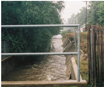
stormwater wall collapse
